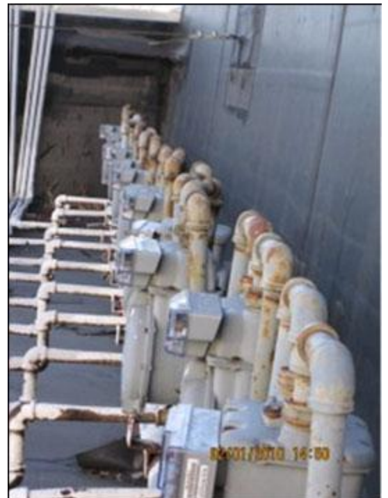
Electricity meters at the Cameron Butcher building in downtown Colorado Springs.
